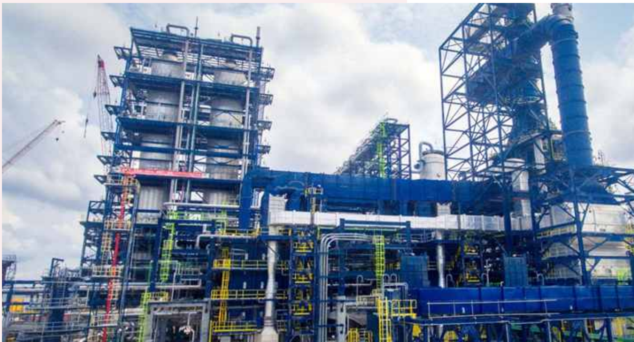
Dangote Refinery Photo Credit: The Guardian
